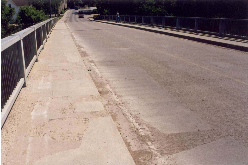
Figure 5 Bridge Street Showing Extensive Patches in Deck and Sidewalk
