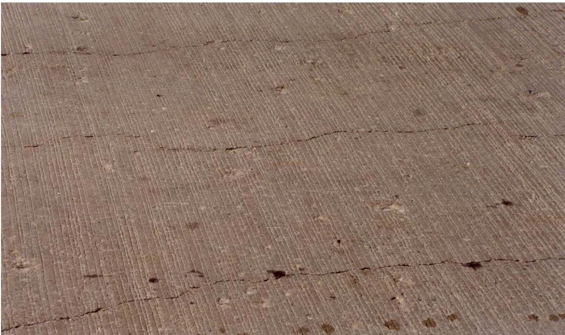
Figure 4 Victoria Street Bridge Showing Cracks in Concrete Deck (1998)
