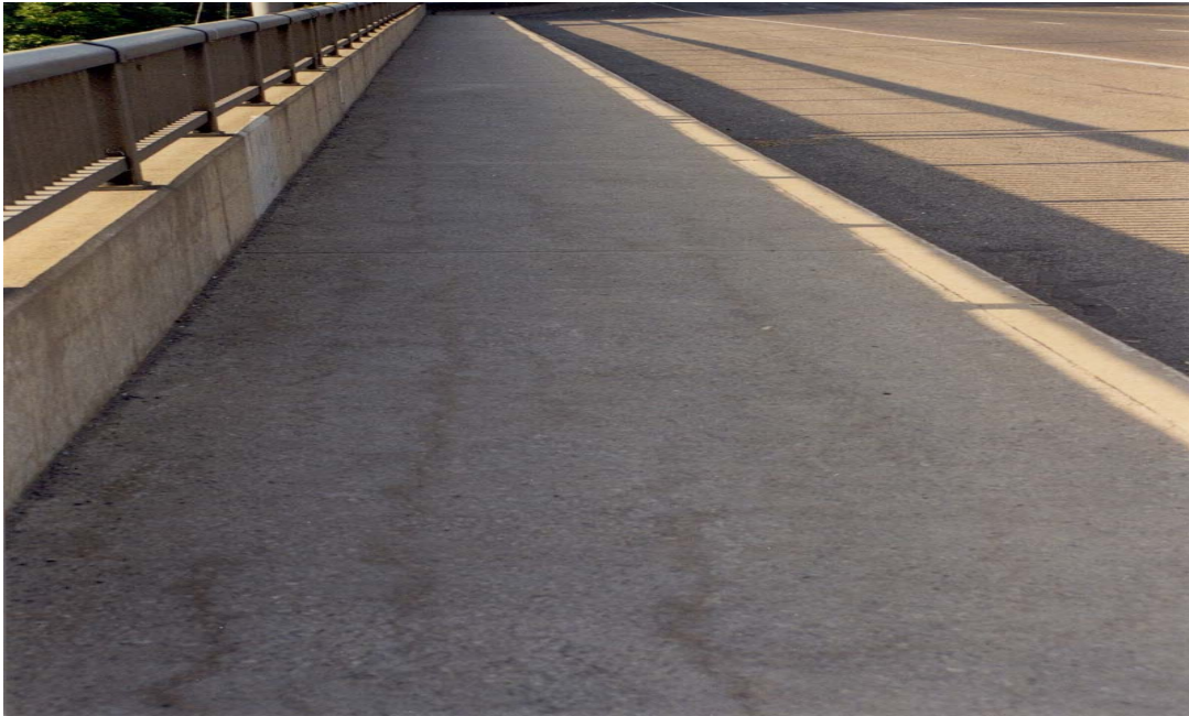
Figure 6 Bathurst Street Showing Cracks and Staining in East Sidewalks
